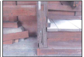
④縁束腐朽
